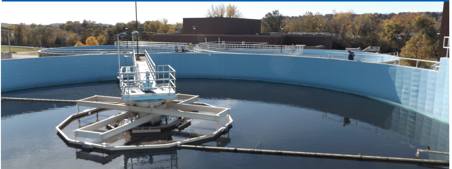
Mankato Wastewater Treatment Plant
