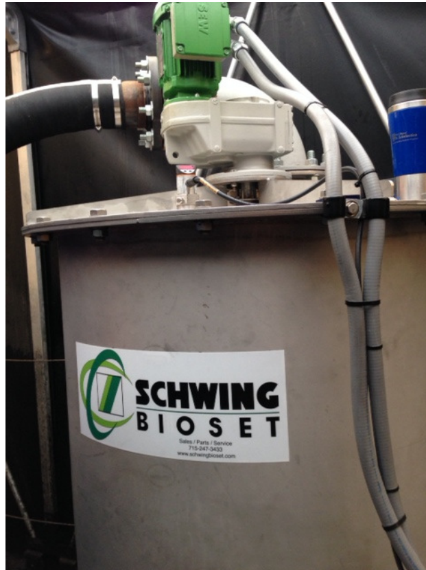
Floc Mixing Tank Setup Schwing Bioset Pilot
