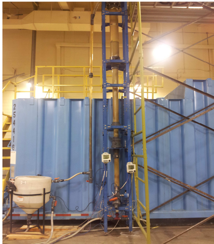
Figure 3: Ostara's Pearl® 5 pilot unit at The City of St. Cloud WWTF
