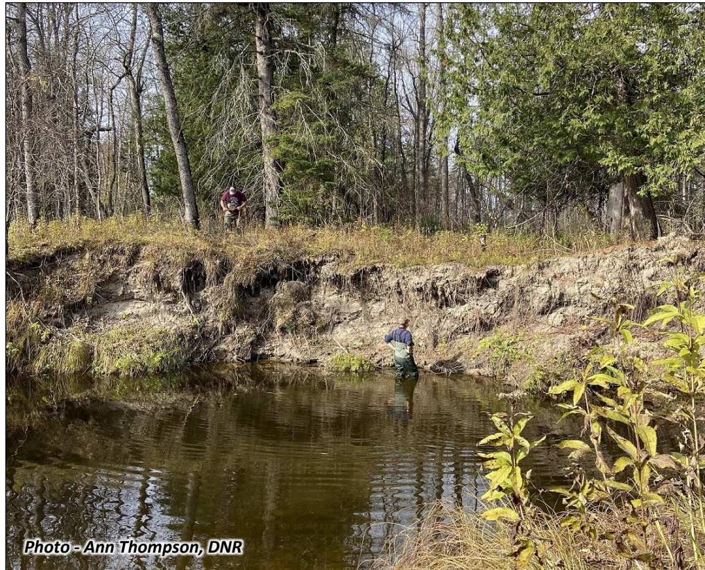
Figure 15. Actively eroding raw vertical stream bank within the geomorphology study reach.
