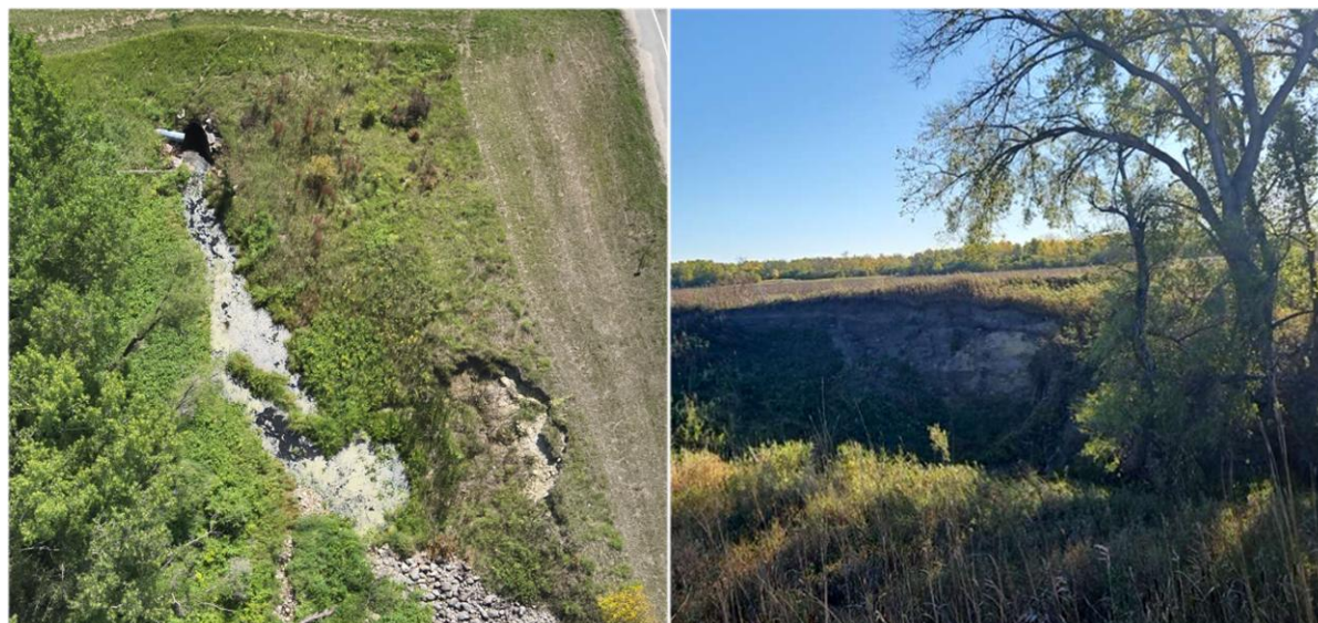
Figure 10. Images of bank erosion along Judicial Ditch 60 (AUID 09020303-570), including Station 23RD101 on June 13, 2012 (left) and near Site S017-320 on October 8, 2025 (right).
