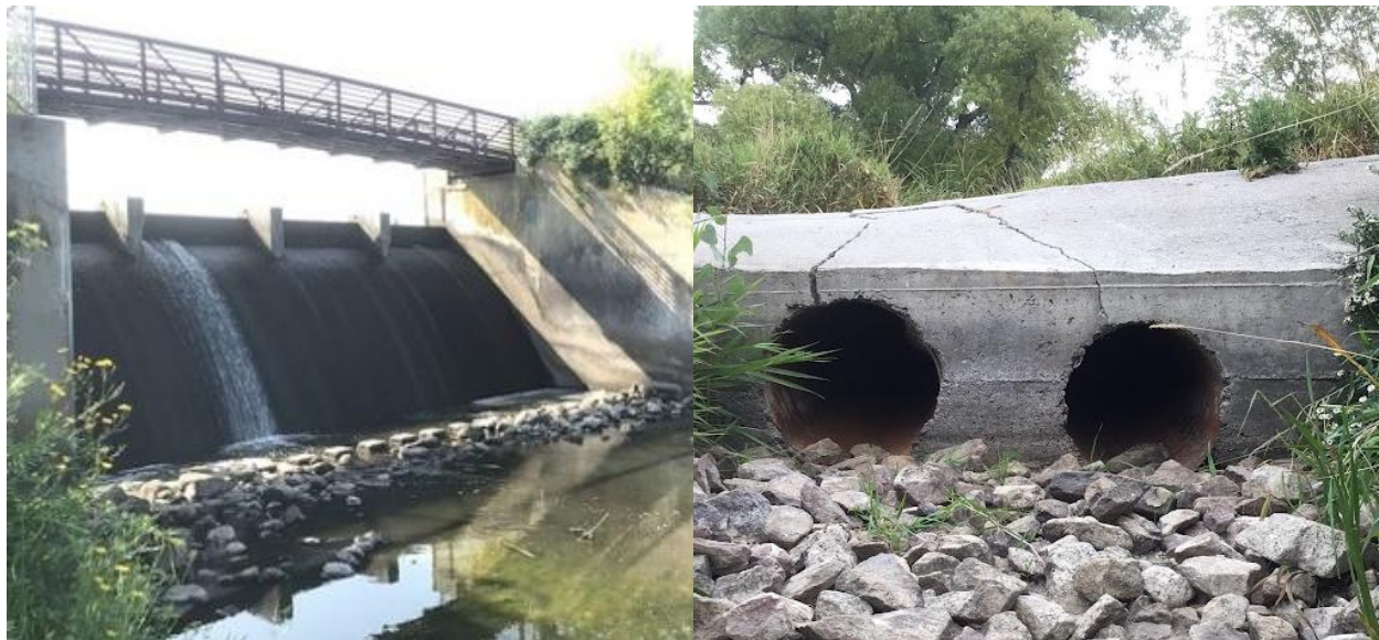
Figure 1. Images of connectivity barriers, including the Mustinka River Dam located at the outlet of the Mustinka Flowage (Pine Ridge Park) along the Mustinka River (09020102-582) on July 18, 2023 (left) and perched culverts associated with a Texas-style crossing located upstream of the 170th St crossing along Unnamed Creek (09020102-563) on September 14, 2023 (right).
