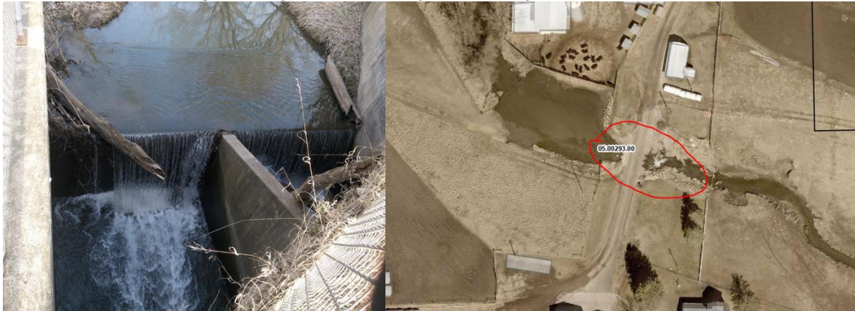
Figure 9. Two connectivity barriers are currently identified on Gorman Creek. Left: A 6 ft drop/box culvert barrier at Hwy 61, downstream of 10LM030. Right: velocity/culvert barrier at private drive, upstream of 10LM030.
