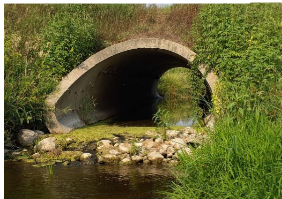
Figure 35. Perched culvert at 10MN083 (8/2/21).
