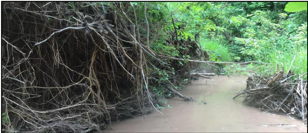
Figure 4. Steep, high, and severely eroded streambanks along Deer Creek.
