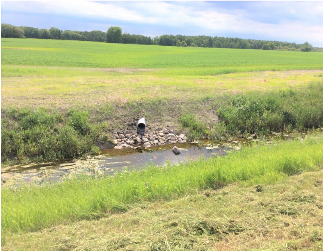
Figure 2. Recently installed side water inlet by Pennington Soil and Water Conservation District.
