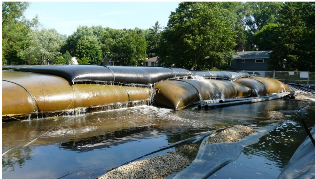
Geo-fabric bags containing stormwater sediment during the de-water phase of the project. Sediment is contained in the bags and filtered water is returned to the stormwater pond.
