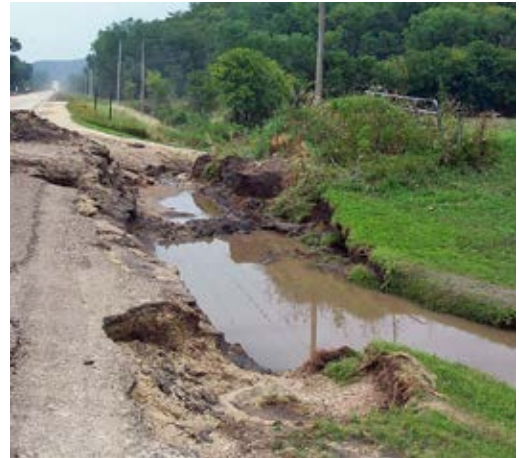
A road near Elba, Minnesota, was damaged by flashfloods in August 2007.
