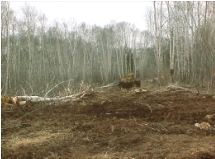
Logging a new Cook County housing development access road near Sugar Loaf Cove. Photo : Courtesy Jesse Anderson
