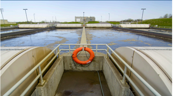
Buffalo Wastewater Treatment Plant
