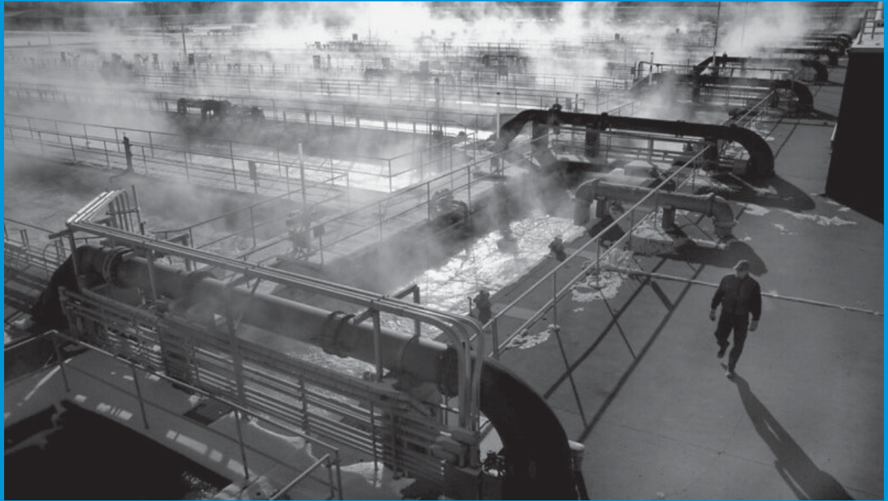
Metropolitan Wastewater Treatment Plant – St. Paul, MN
