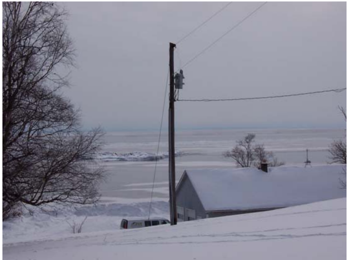
Figure 2. Example of a high priority suspect transformer in the CLP service area.
