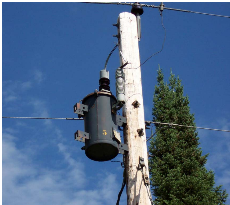
Photo credit: Scott Bohling, MPCA - a suspect transformer in the Lake Country Power service area
