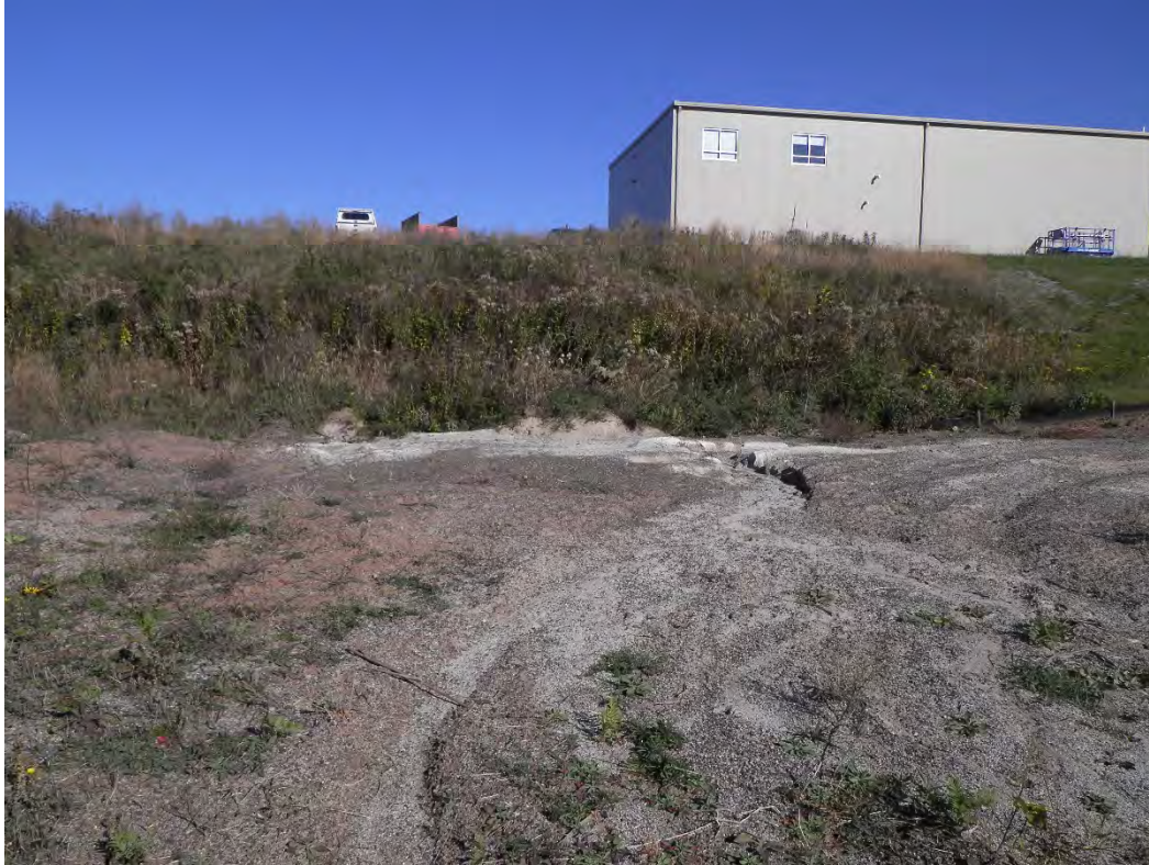
Stryker Bay hillside minor erosion, view north
