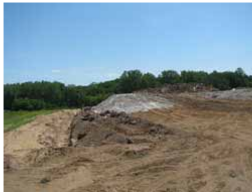
Northeast corner of landfill looking east. Waste stockpile located on top of existing landfill cover. Grey color is a spray-on product to seal surface, to reduce blowing litter and odor.
