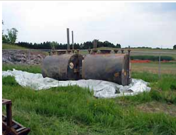
Old storage tanks unearthed from the landfill will be taken off-site for recycling and/or disposal if possible.
