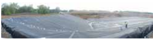
Panorama of first two layers of plastic liner installed and in the process of being tested for leak.
