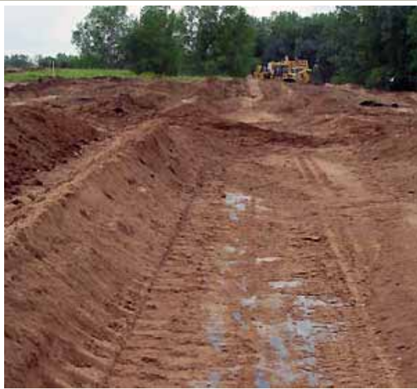
Cover soils have been removed, exposing the synthetic membrane that forms part of the landfill's existing cover system.
