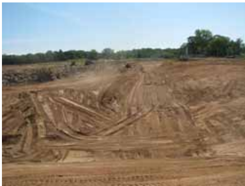
Cell A excavation looking east. South portion at final bottom elevation (not in groundwater). Contractor is excavating waste in north portion.
