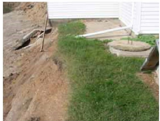
Washed away SSTS in eroded stream bank
