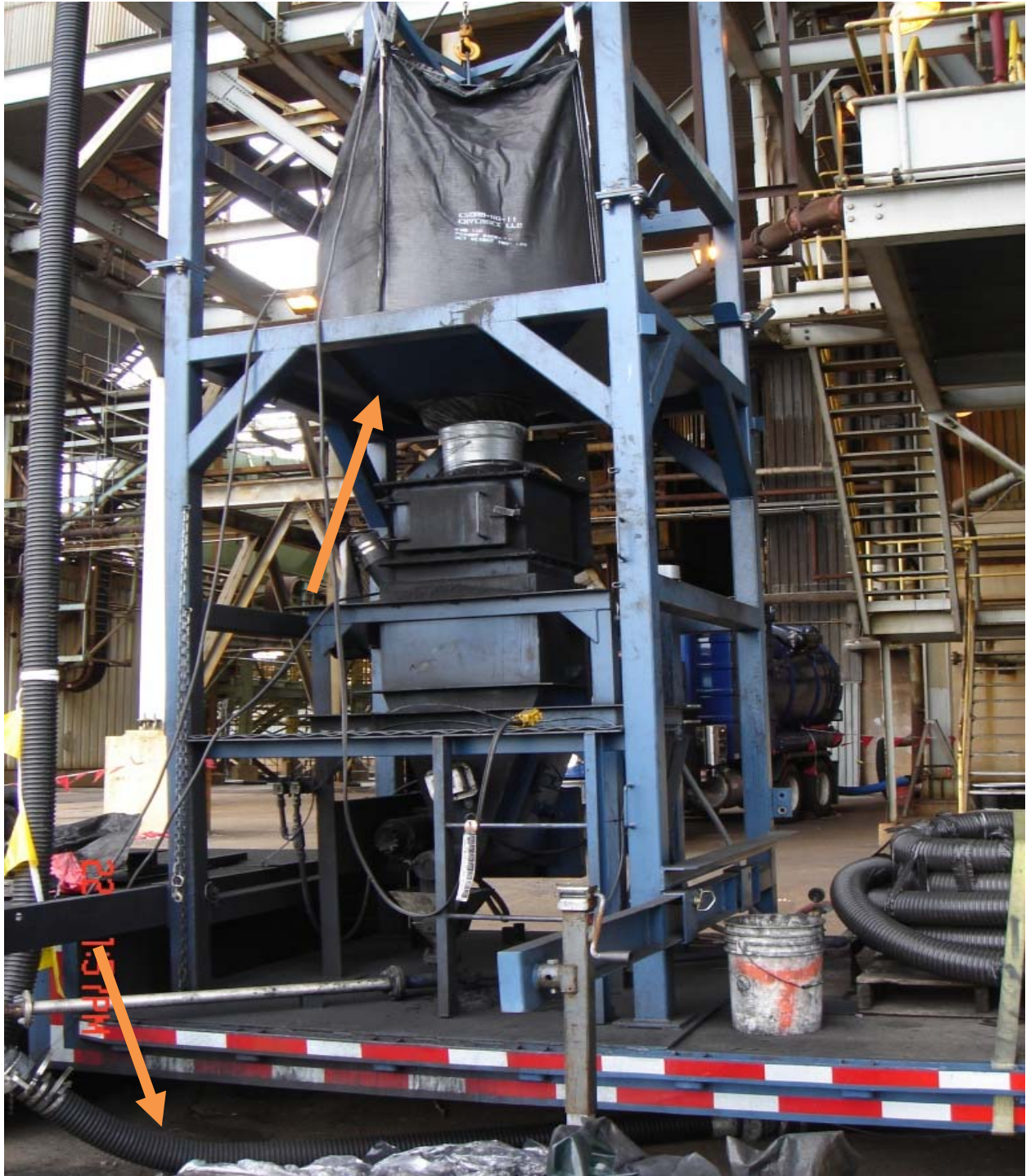
Figure 1. A close-up photo of the sorbent bulk-bag handling system. The bulk bag is placed on the top (upper arrow). The discharge pipe below (lower arrow) comes from the educator and is attached to a hose that connects to the distributors and injection lances.
