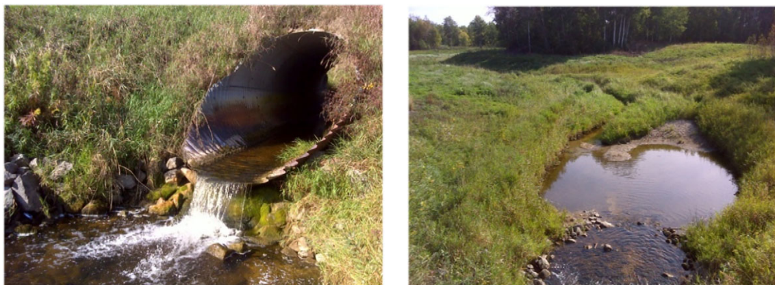
Figure 9. Photos of a perched culvert (left) and its associated plunge pool (right) at the CR 61 crossing along AUID 501.
