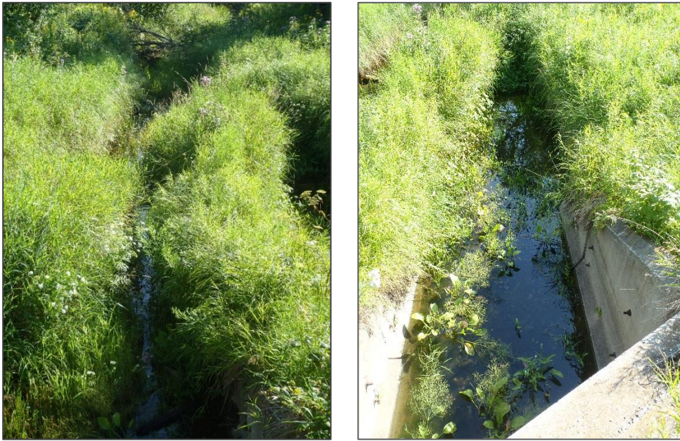
Photo 8. Perry Creek at Buckeye Road, August 3, 2016, looking downstream. Of the paired culverts at this crossing, the left photo is the culvert that carries more of the low flow. The right photo (and right culvert) is a bit out of the channel/thalweg and has accumulated some sediment below the outfall. Emergent aquatic vegetation is growing inside the culvert (very rarely observed), suggesting frequent low flow volumes or stagnant conditions (as it was here).
