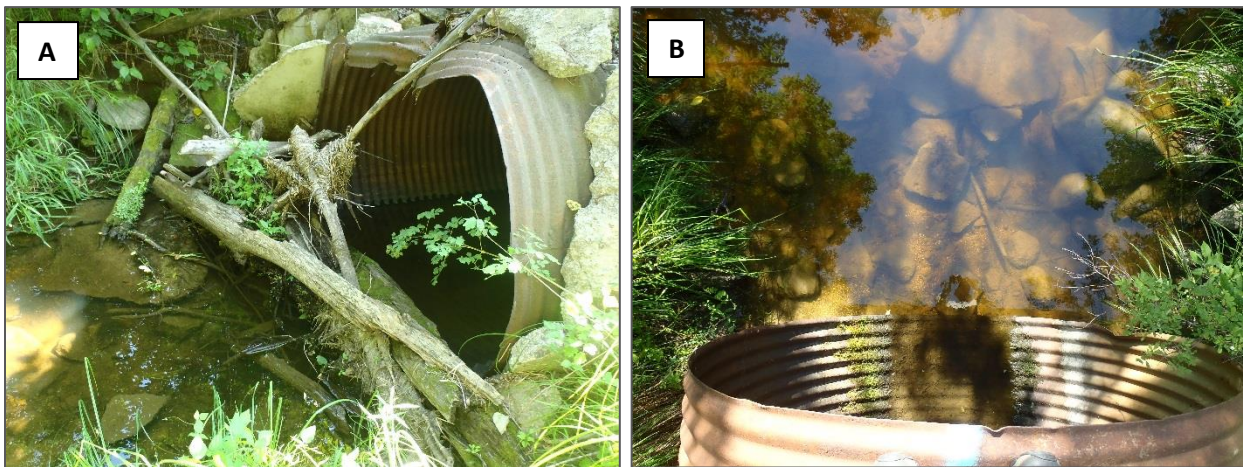
Photo 10. August 3, 2016. A. Upstream end of culvert on private field-access road, showing debris accumulation, B. Downstream end of culvert showing a nearly-perched condition.
