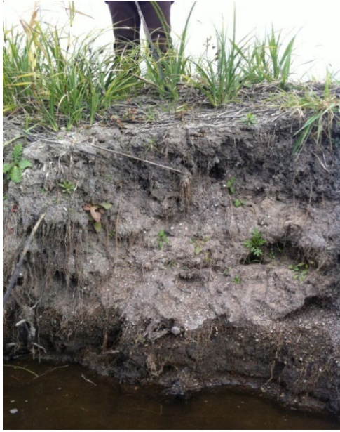
Photo 10. Bank erosion within the geomorphology study reach. The banks are a significant source of sediment to the channel with the current hydrological regime. Riparian vegetation roots are inadequate to hold the streambank soil. The granular soil material (sand and small gravel) below the 12-inch topsoil layer is relatively susceptible to erosion by stream currents.
