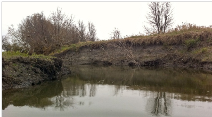
Photo 13. Bank erosion on both sides of river at a bend signals downcutting (incision) of the channel. The erosion of banks are contributing to the turbidity and bedded sediment problems.
