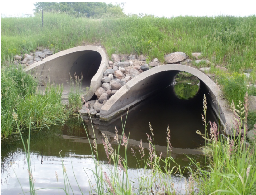
Photo 16. CSAH 7 culverts are very well-designed for fish passage (one culvert carries baseflow, and one culvert set at the floodplain elevation). This design maintains proper stream geomorphology, and reduces erosion of the streambed and banks.
