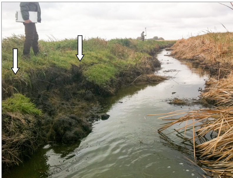
Photo 9. Bank destabilization within study reach EOR-51. Arrows point to formation of fissures, which will likely lead to a sizeable section of bank collapsing into the creek, as happened between the arrows. The roots of the short grasses here are insufficient to structurally hold the sharply-angled bank.
