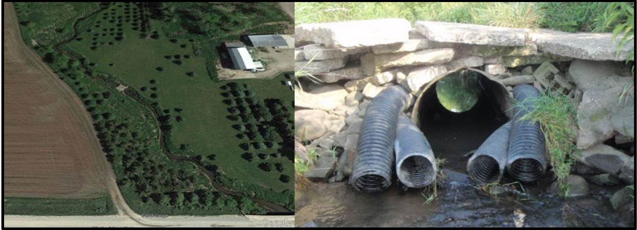
Figure 15: Photos of culvert at station 15CD012. During fish sampling, it was noted that “there is a culvert in the middle of the reach that could act as a fish barrier at times of low flow or drought, but during normal flow it looks like fish should be able to pass.” The photo on the left is courtesy of Google Earth.
