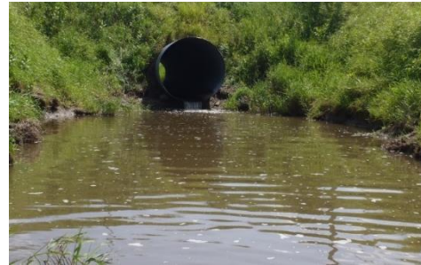
Figure 178. Perched culvert at site 14MN080 (July 19, 2014)
