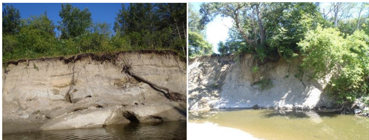
Figure 81. (Left) Eroded bank at site 14MN061, (Right) Eroded bank at site 14MN082.
