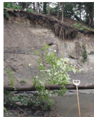
Figure 193. Severe bank erosion at site 00MN007 (August 19, 2014)
