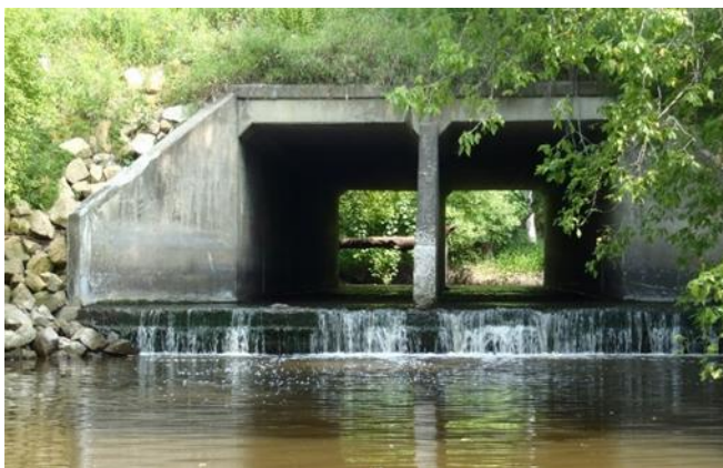
Figure 260. Perched culvert at site (August 7 2014)
