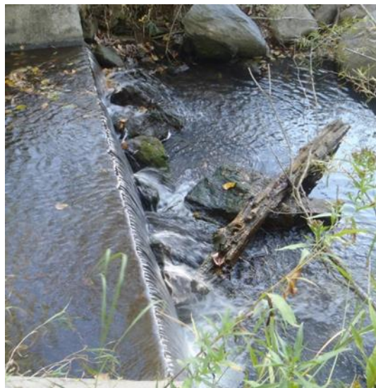
Figure 195. Perched culvert at site 00MN007 (September 26, 2013)
