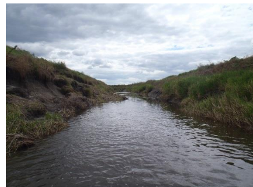
Figure 59. Bank erosion at site 14MN052 (July 15, 2014)
