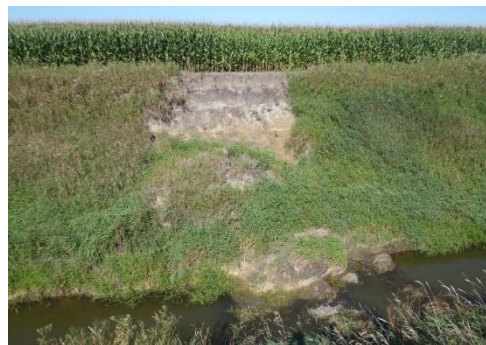
Figure 172. Erosion at site 14MN081 (August 12, 2014)
