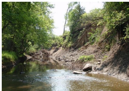
Figure 223. Heavy bank erosion at site 14MN090 (August 18, 2014)
