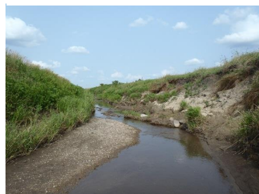
Figure 72. Erosion at site 14MN060 (July 30, 2014)
