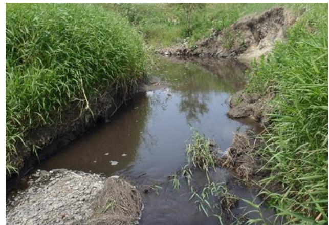
Figure 67. Erosion and sediment at site 14MN083 (July 30, 2014)
