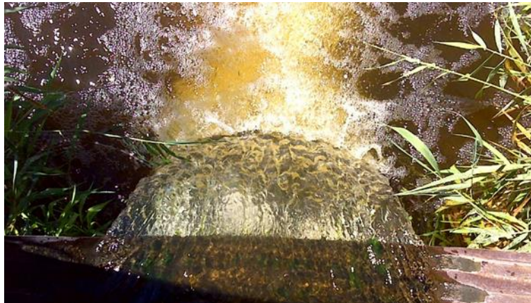
Figure 277. Perched culvert at site 14MN030 (August 31, 2016)
