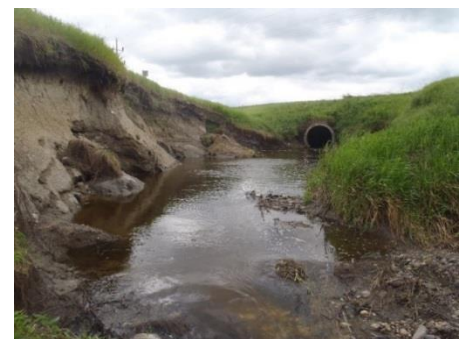
Figure 91. Severe erosion at site 14MN220 (July 14, 2014)
