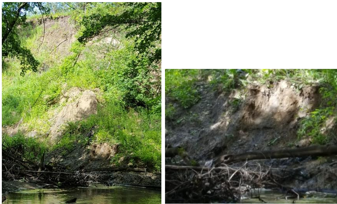
Figure 232. Erosion at site 99MN004 (July 7, 2016)
