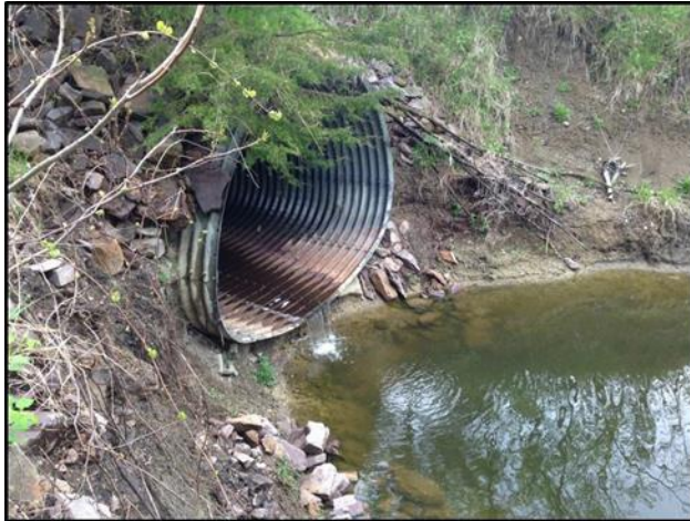
Figure 46. Perched culvert. Photo credit DNR
