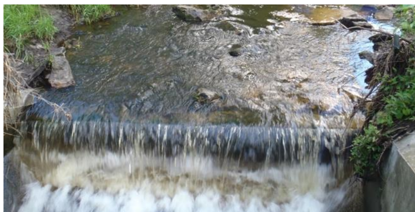
Figure 214. Perched culvert at site 01MN058
