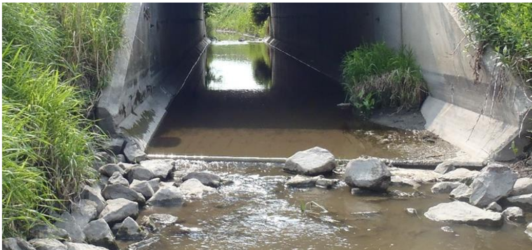
Figure 75. Perched culvert at site 14MN060 (July 30, 2014)
