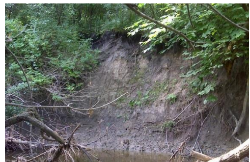
Figure 291. Erosion along Bluff Creek (July 5, 2016)
