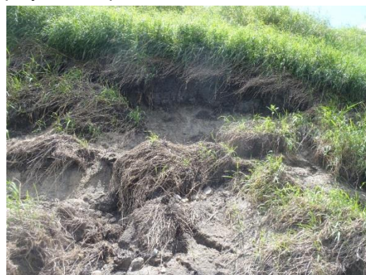
Figure 29. Eroded stream bank at site 14MN071. (July 16, 2014)
