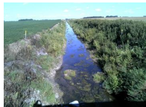
Figure 9. Poor sinuosity at site 07MN083 (August 20, 2018).
