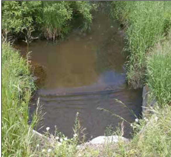
Photo 9. The upstream side of the culvert at 365 th Street (07UM019). The lip of the culvert is up off the bottom of the stream bed and velocity can be seen picking up immediately upon reaching the culvert.
