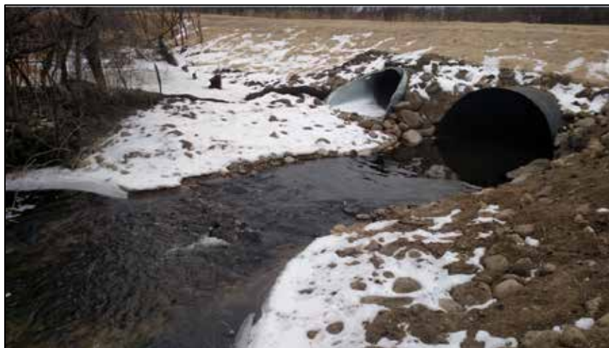
Photo 20. Downstream side of new culverts on Sucker Creek at 650 th Avenue, southeast of Litchfield. The main culvert is properly sized and set at the appropriate elevation to allow natural continuity of the stream through the culvert. The floodplain culvert allows for high streamflow to pass and protect the roadway.
