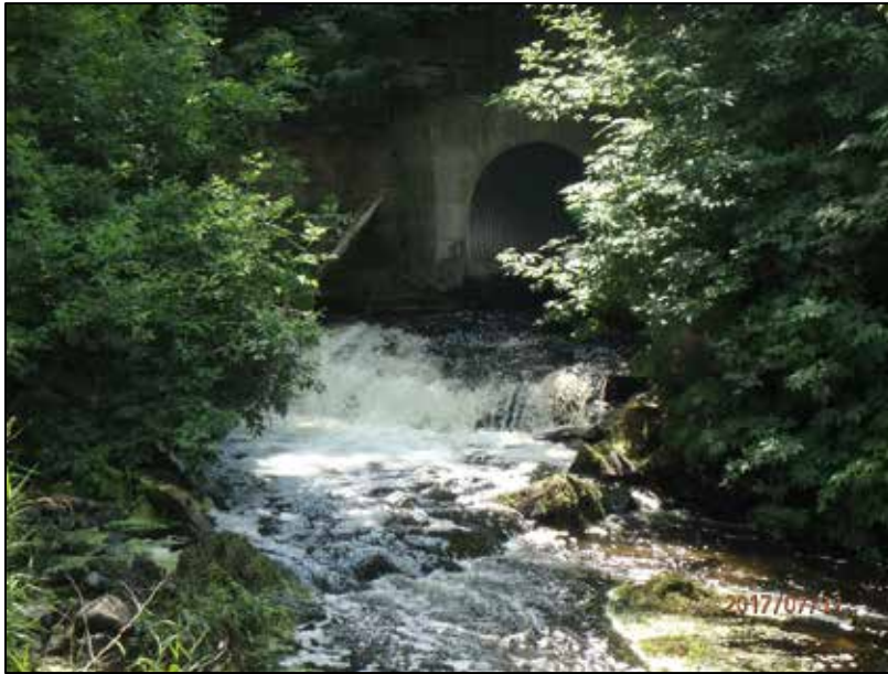
Figure 80. Perched culvert below the railroad grade, located 0.5 miles upstream of U.S. Highway 12 on Grove Creek, creating a fish passage barrier.
