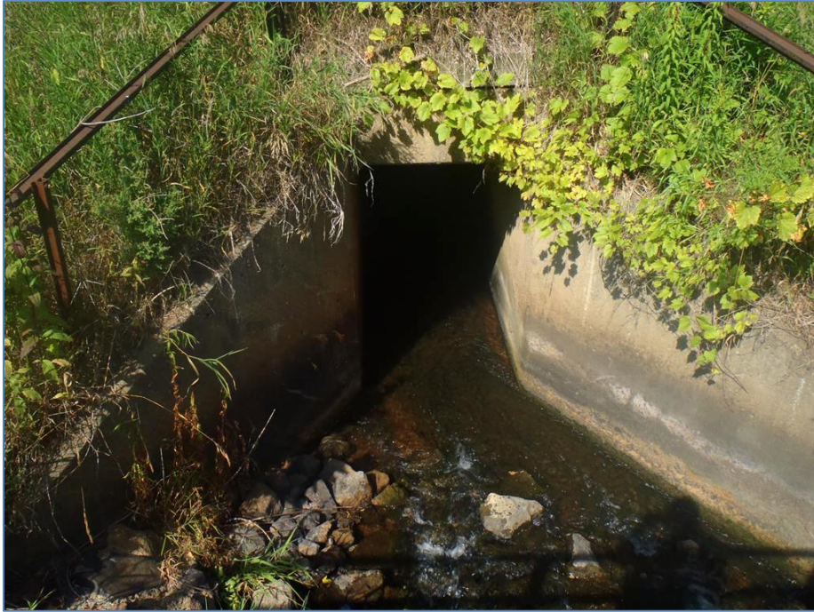
Figure 55. Inlet of Stearns County CSAH75 culvert.
