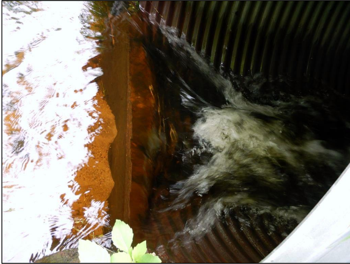
Figure 41. Inlet of Great River Rd. culvert. Photo taken 7/13/2018. Wooden board laying across opening is creating a perched inlet and excessive velocity barrier to fish passage.
