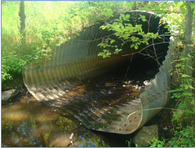
Figure 60. Inlet of culvert at Stearns CR160, just upstream of 07UM101. There are two CR160 crossings with the South Fork of the Watab River; this is the one furthest east.
