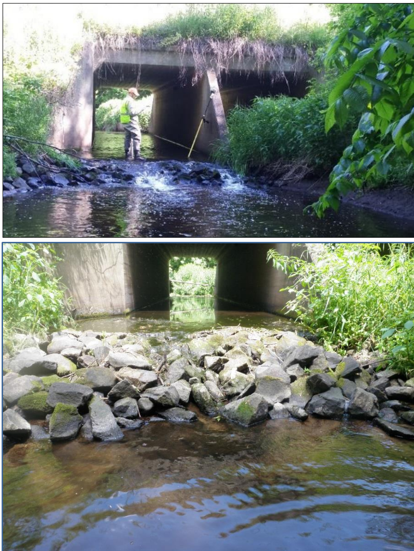
Figure 94. Pictures of the Zuleger Creek crossing with Benton County Road 12, illustrating the barrier to fish passage.
