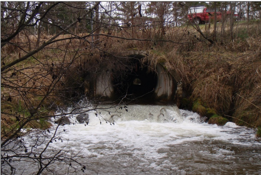
Photo 4. Perched culvert at Sugar Hills Road is an impassible barrier to fish migration.
