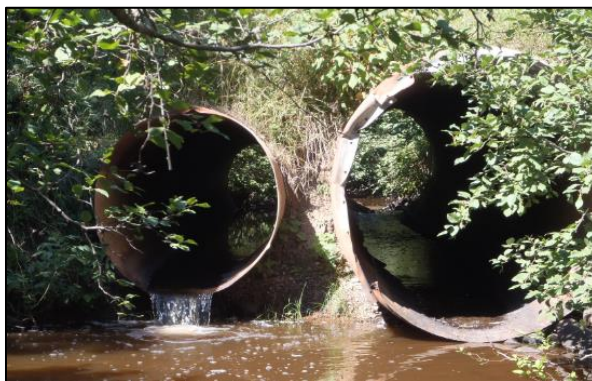
Figure 33. Undersized and perched culverts at Camp 20 Rd (CR 70).
