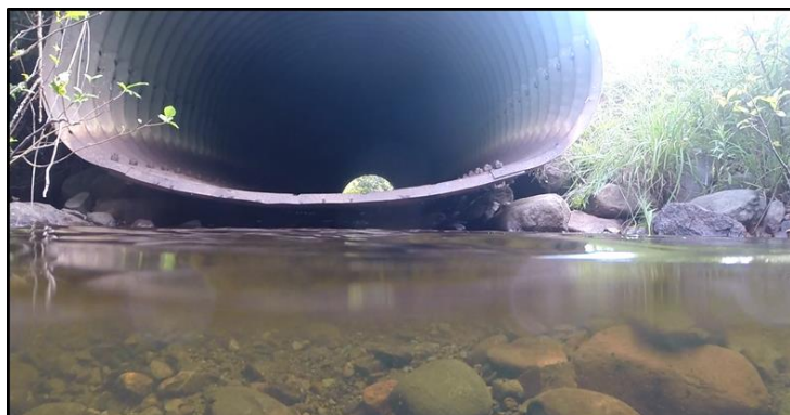
Figure 60. Water level view of perched and undersized road culvert at Cook County HWY 1. The culvert is fractured in numerous locations along its length beneath the road allowing water to flow freely beneath the road grade.
