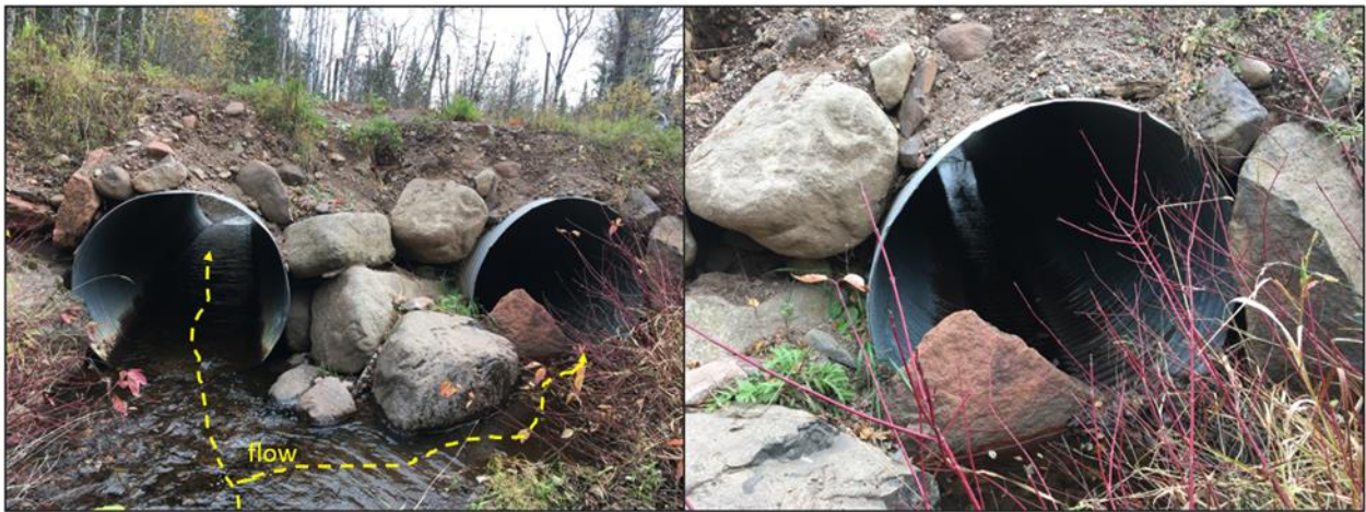
Figure 76. Looking downstream at Cooper Rd crossing of Lindstrom Creek. Blockages of the river-right culvert disrupt sediment transport and alter current velocities and water depth and velocity within the structures.
