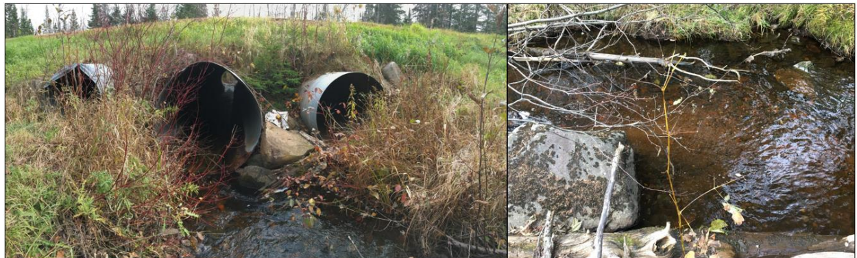
Figure 77. Perched and improperly set culverts at the Cooper Rd crossing create a partial barrier to fish passage (left), while a span bridge located just downstream allows full fish passage and helps maintain channel stability.
