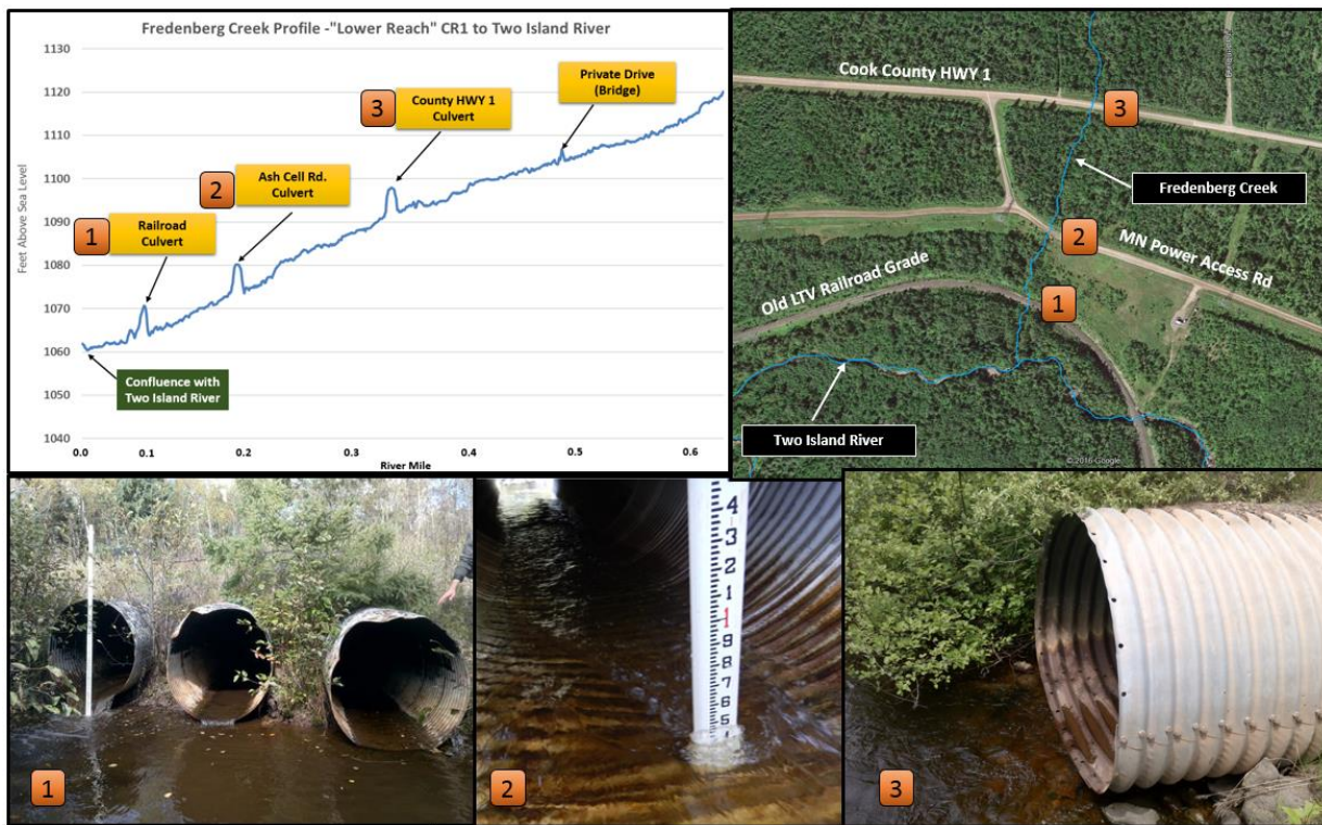
Figure 59. Longitudinal profile of Fredenberg Creek and location of the three undersized and poorly installed road culverts that act as partial to full barriers to the migration of wild Brook Trout, other non-game fish species, and terrestrial and semi-aquatic species that use riparian corridor habitats (e.g. turtles, otters).
