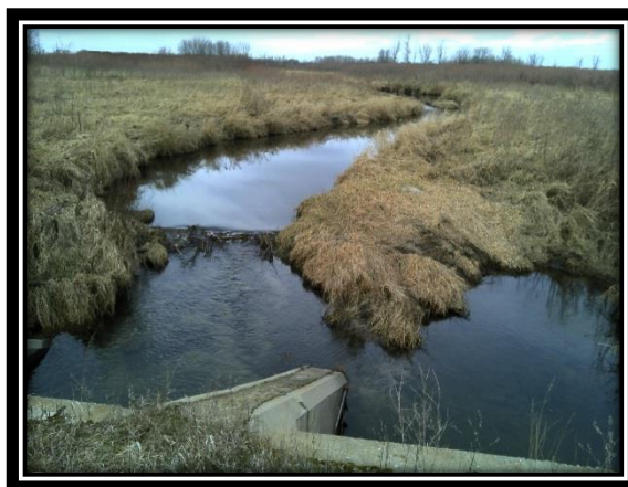
Figure 2 - Poorly Aligned Culvert on Pine Creek.
