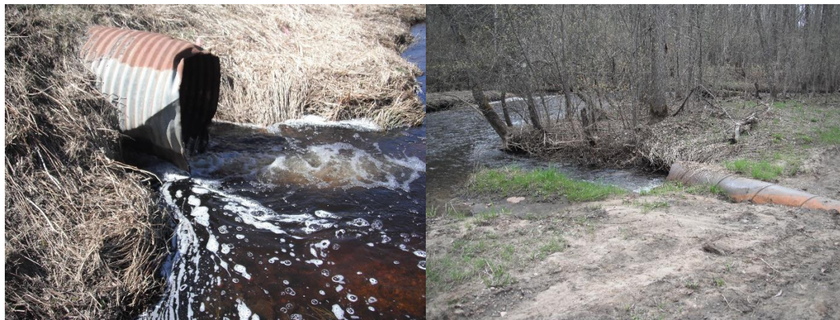
Figure 33. Examples of culvert issues in the MRGRW (Rian Reed 2019)
