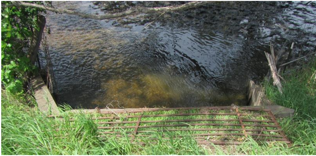
Figure 43. Cattle gate connected to the CR 45 culvert, using the culvert for cattle passage under CR 45.
