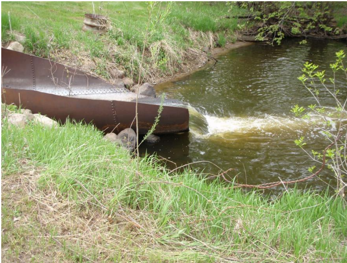
Figure 66. Perched culvert off 57th Street SE.
