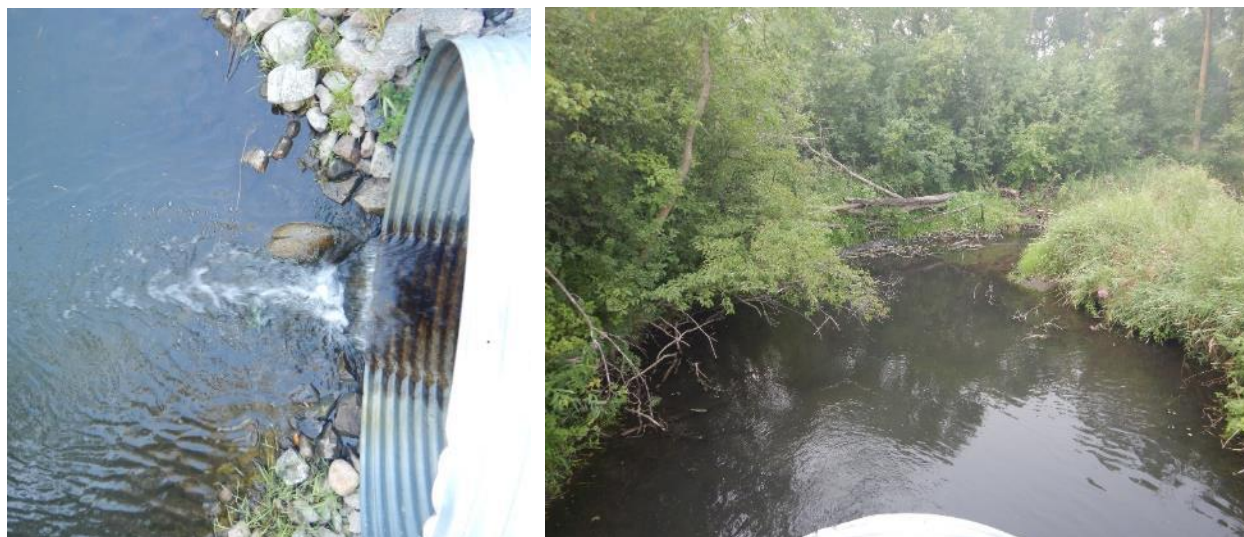
Figure 45. Perched culvert off 160th St.
