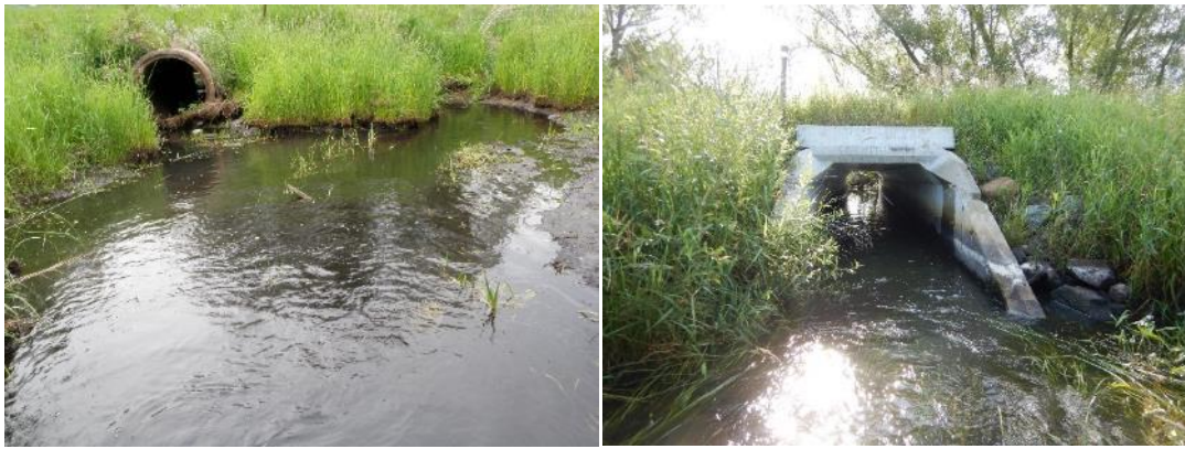
Figure 48. Culvert crossing replacement at the 45 th Ave SE crossing from June 2009 to July 2019.
