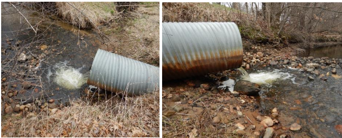
Figure 75. Perched culverts on small tributary streams flowing into the Snake River.
