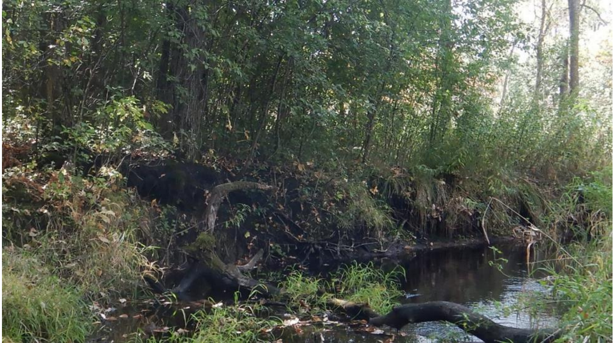
Figure 39. Eroding stream bank on the -564 reach of Threemile Creek.
