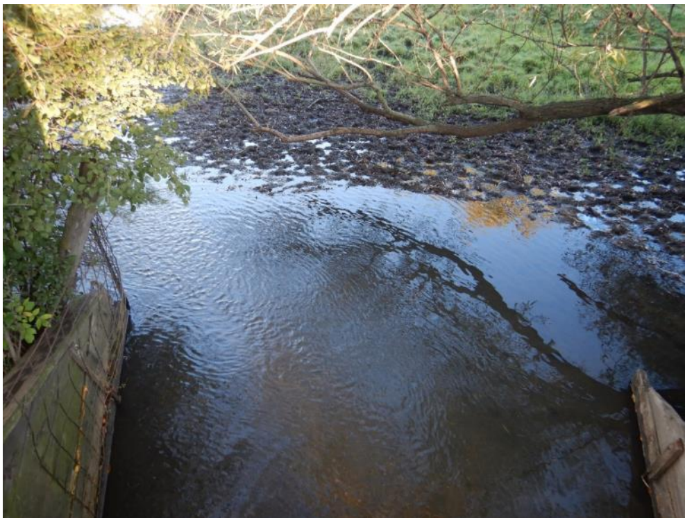
Figure 42. Channel erosion caused by cattle trampling, upstream of CR 45.
