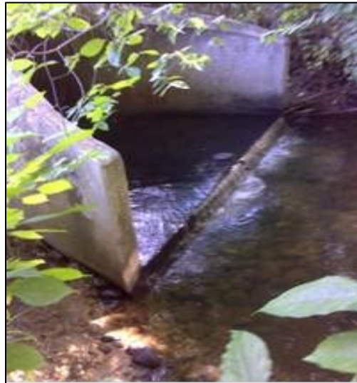
Figure 12. Downstream portion of culvert under CSAH 14 on the Tributary to Lake Miliona.
