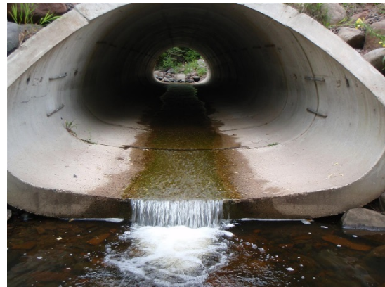
Figure 48. Perched culvert, Woods Creek at Cook County Road 58.
