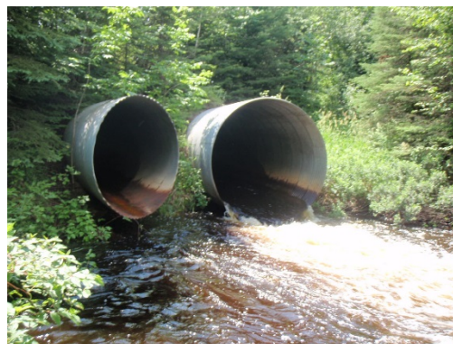
Figure 69. Perched culvert on Hockamin Creek, at the Heffelfinger Road.
