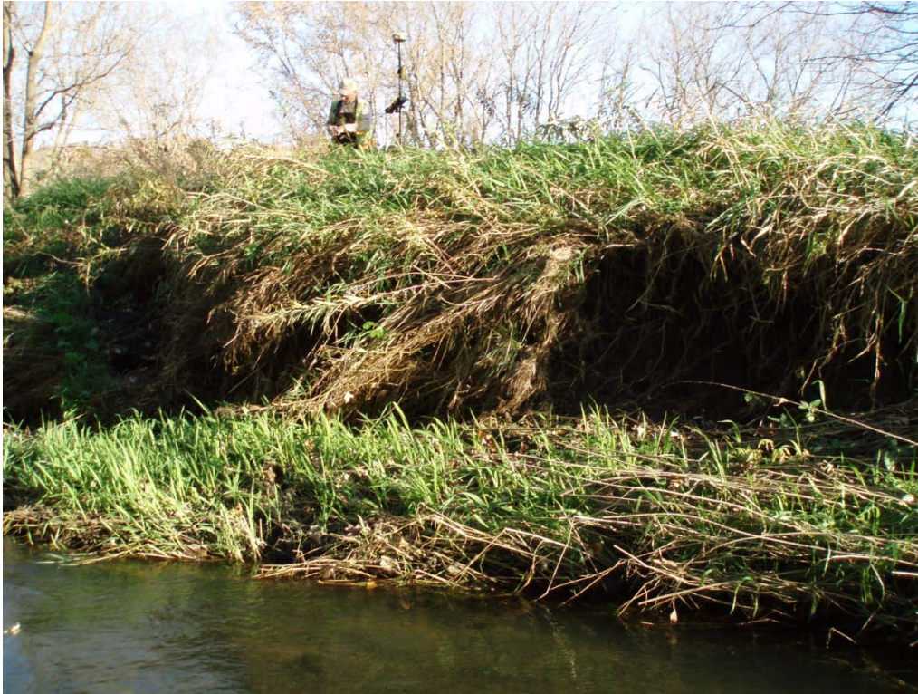
Photo 4-3. Bank erosion at Site 4.
