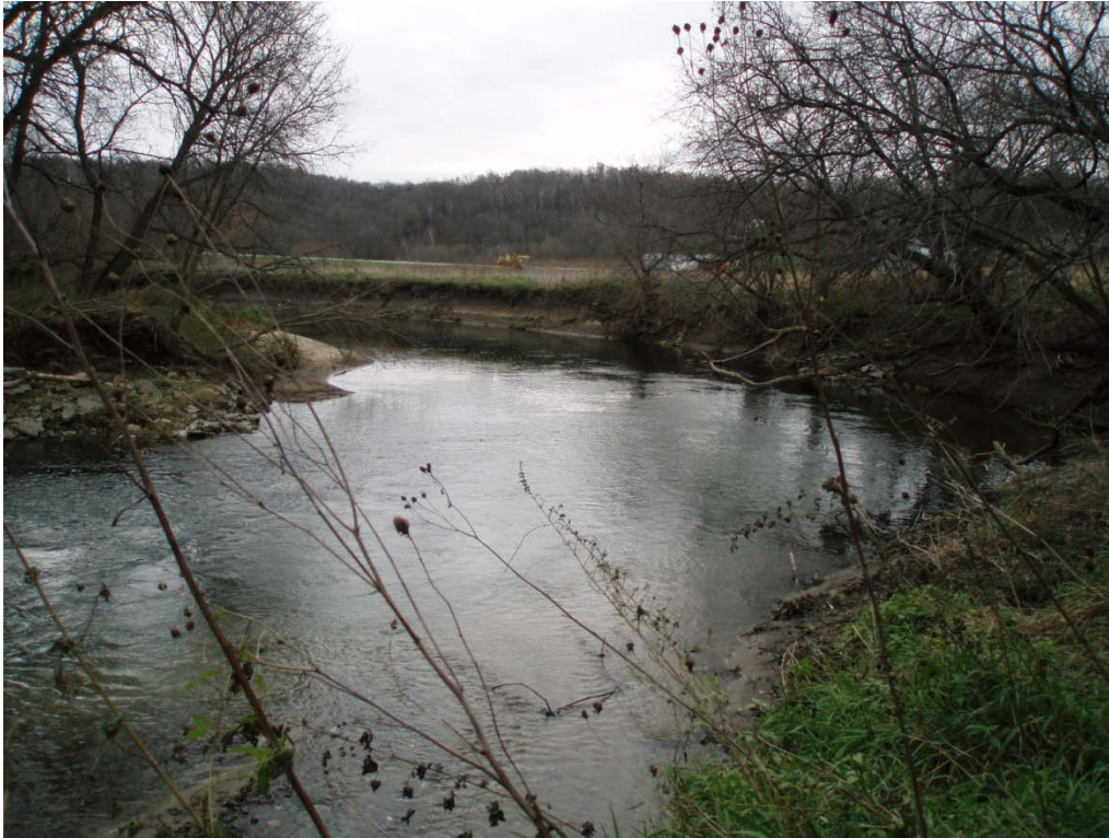
Photo 7-3. Bank erosion at Site 7
