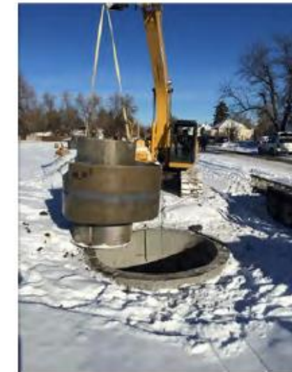
Hydrodynamic Separator (CDS Stormwater Treatment)
