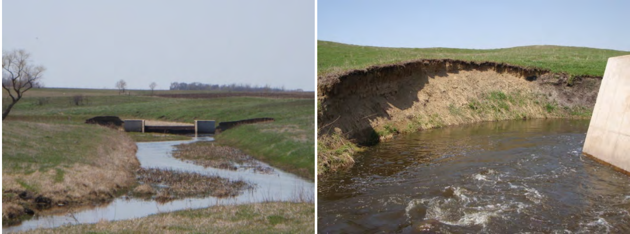
Figure 33. Impoundment on Dry Wood Creek no longer functioning, May 5, 2008
