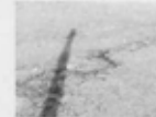
Surface discharge from non-compliant septic system that would be considered an ITPHS.
