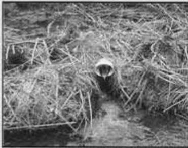
Septic systems that illegally discharge to the river are a source of fecal contamination.
