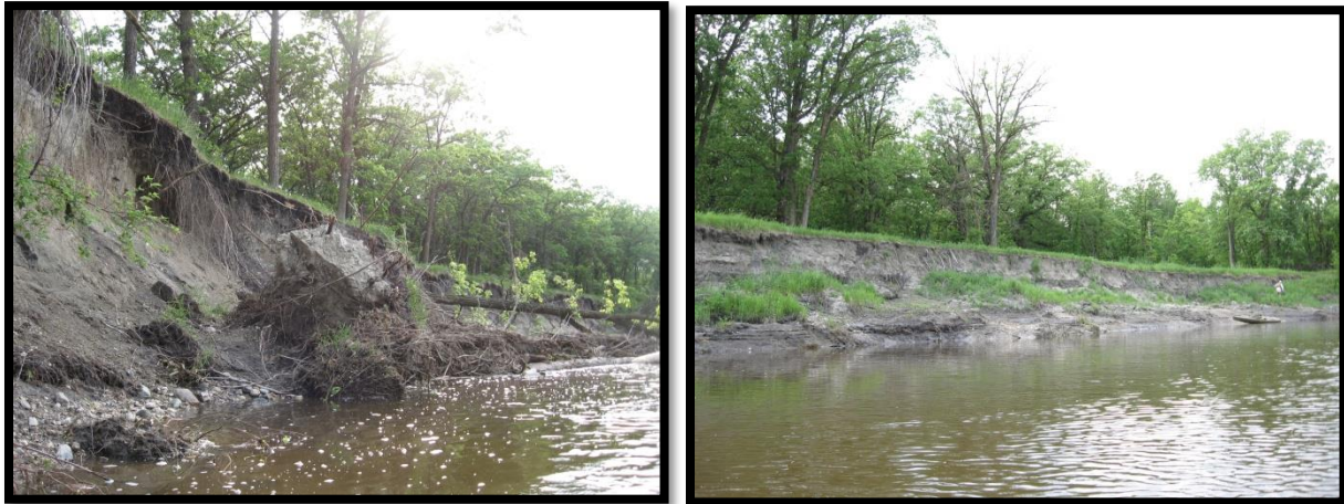
Figure 8-2. Photos of actively eroding streambanks along the Thief River
