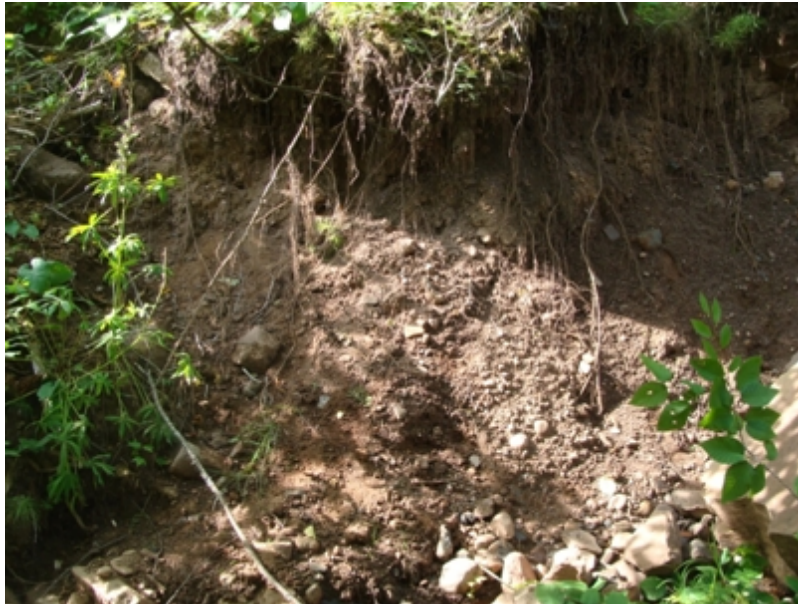
Figure 12. Forested ravine eroding bank
