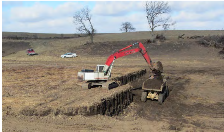
E3 flood control structure clean out in Crystal Creek Watershed. 20,000 cu. yds. Nov. 2017
