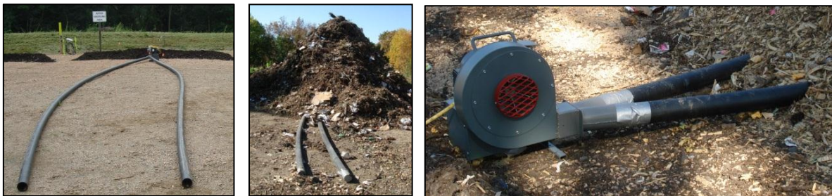
Above (left): Aeration tubes lined up on the pad. Above (middle): Aeration tubes coming out of a pile. Above (right): Blower and aeration tubes entering the pile.
