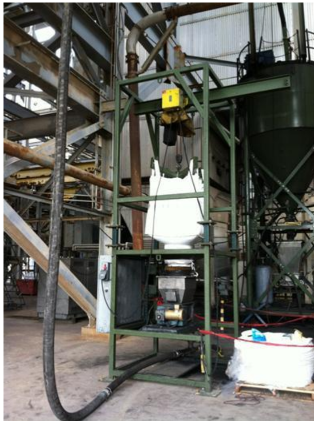
Figure 3. DemoPAC Injection Equipment
