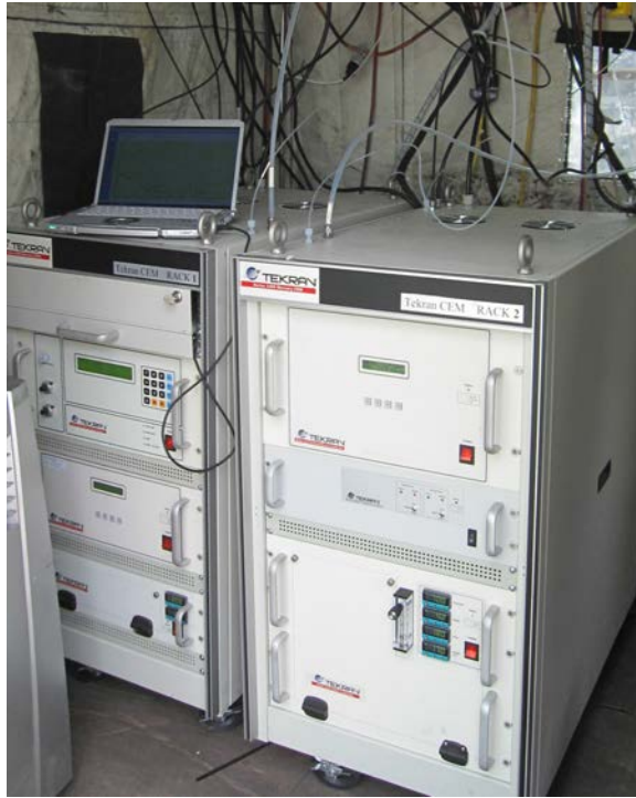
Photograph 3. Tekran Mercury Conversion Module and CEM
