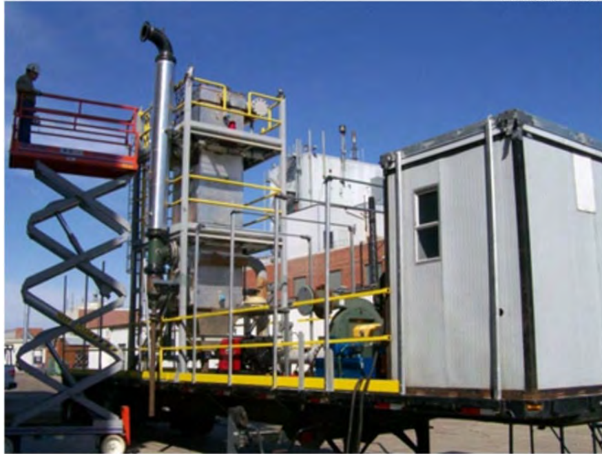
Figure 1. Photograph of the EERC baghouse, trailer, and control room.
