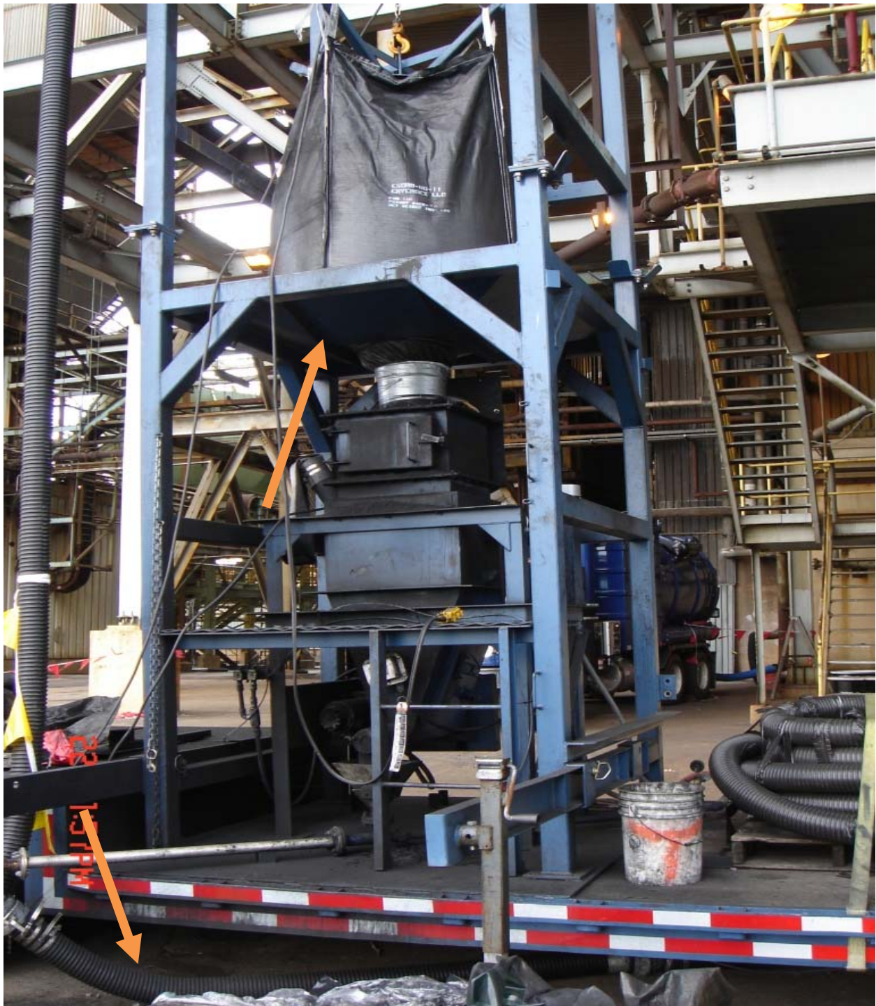
Figure 1. A close-up photo of the sorbent bulk-bag handling system. The bulk bag is placed on the top (upper arrow). The discharge pipe below (lower arrow) comes from the educator and is attached to a hose that connects to the distributors and injection lances.
