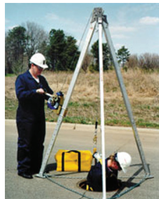
Figure 11-1: Stay safe in confined spaces
