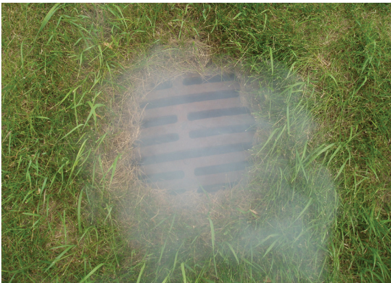
Figure 2-4: Smoke test showing inlet location
