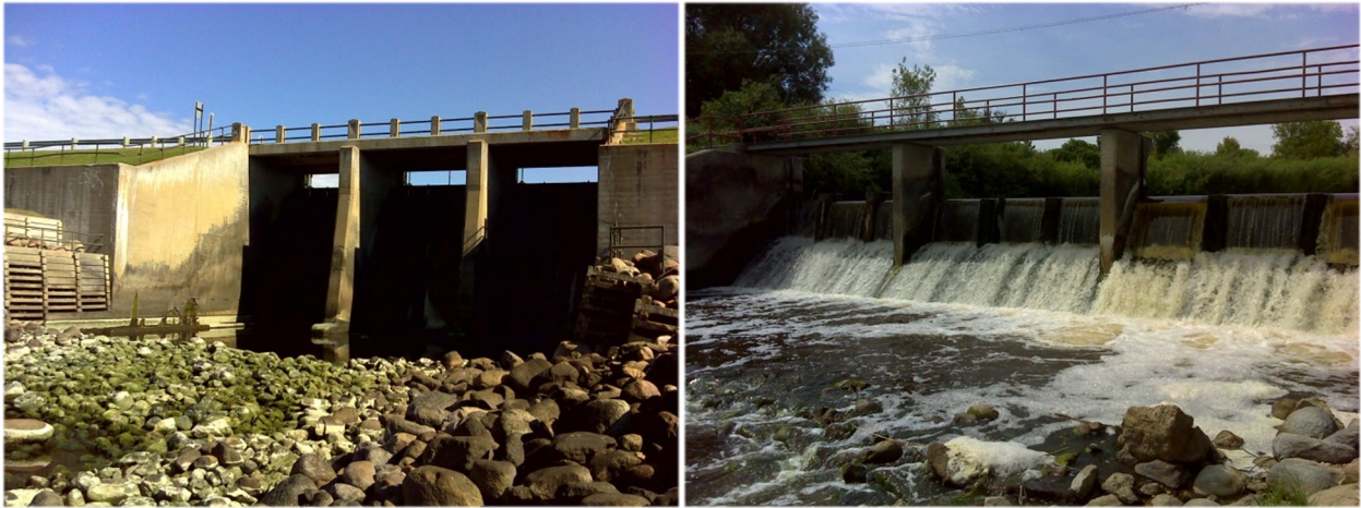
Figure 9. Photos of connectivity barriers along AUID 502, including the Lake Bronson Dam on September 23, 2015 (left) and the Hallock Dam on August 12, 2015 (right).
