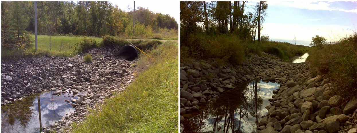
Figure 65. Photos of connectivity barriers affecting AUID 522, including a perched culvert along CR 105 on September 23, 2015 (left) and a rock check dam along CR 105 on September 23, 2015 (right).
