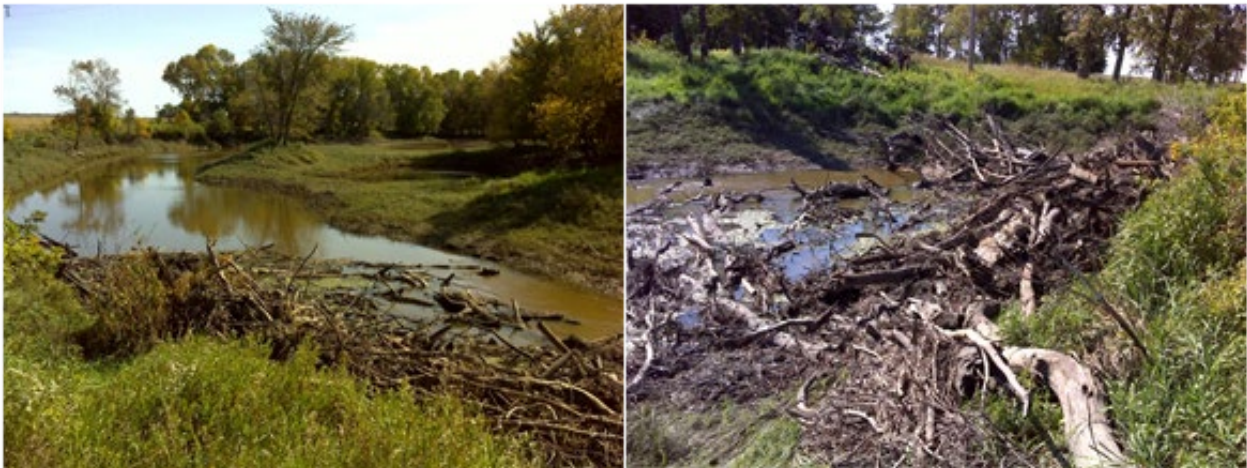
Figure 24. Images of a log jam located at the 330 th Street NW crossing along AUID 502 on September 21, 2016.
