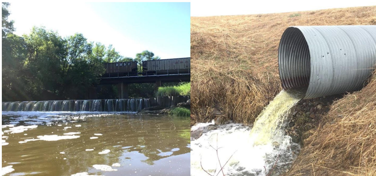
Figure 2. Images of connectivity-related issues, including the Ganz Dam located upstream of the US Highway 10 crossing along the Buffalo River, South Branch (AUID 09020106-503) on August 28, 2019 (left) and a perched culvert located at the 140th Ave crossing along Unnamed Creek (AUID 09020106-576) on April 12, 2021 (right).
