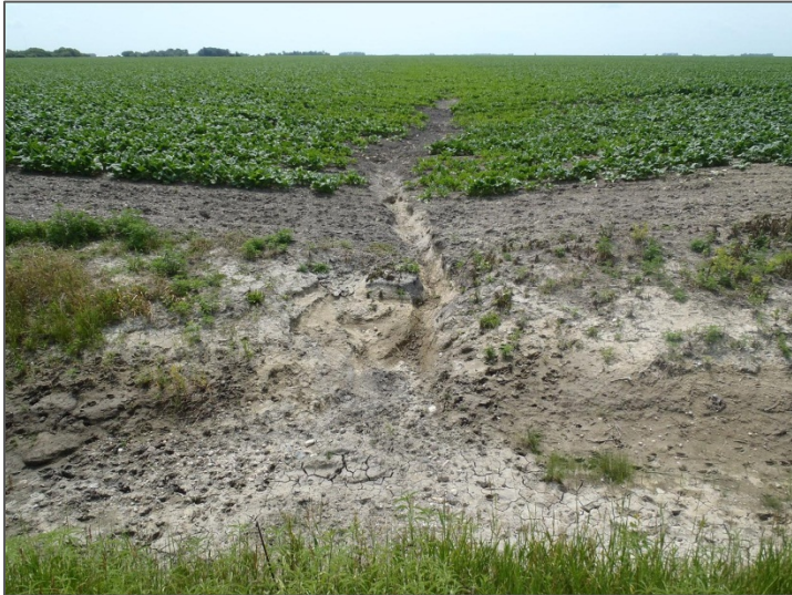
Photo 8. Surface erosion from an unvegetated field swale along State Highway 75. A significant delta of soil has been deposited in the ditch, where it can move downstream farther. There were several of these from this
