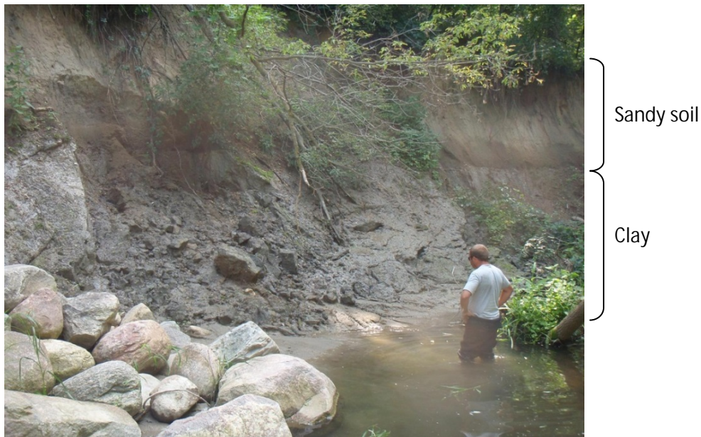
Photo 19. Mass wasting along the channel just downstream of the Township Road 18 crossing. The upper material is sandy, while the lower material is groundwater-saturated clay.
