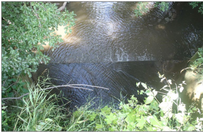
Photo 18. The culvert bottom (a cement apron) is perched above the stream bottom, resulting in a vertical drop in water surface levels of about a foot.
