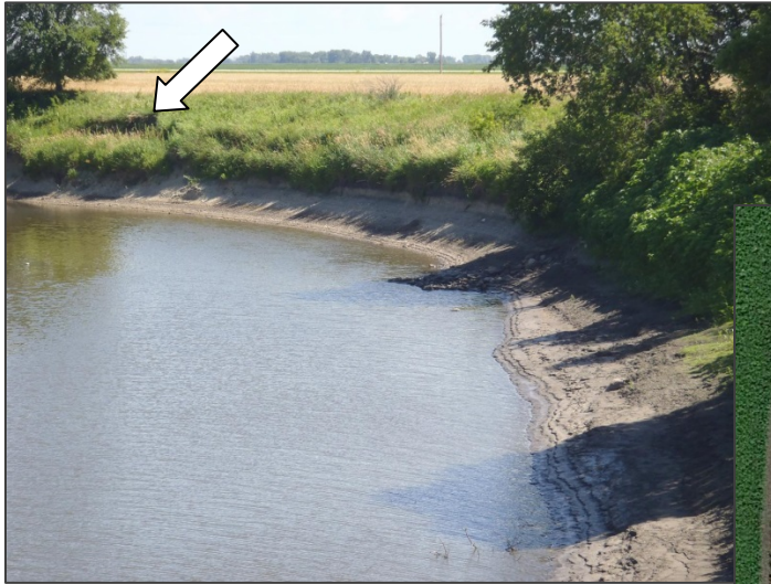
Photo 1. Looking downstream from the CSAH-6 bridge. The arrow points to a large piece of bank material caving into the channel.
