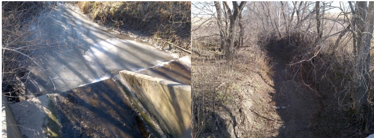
Figure 48: Perched culvert (left) and dry streambed (right) from November 22, 2017, reconnaissance visit; both are located just south of the MN/IA border.
