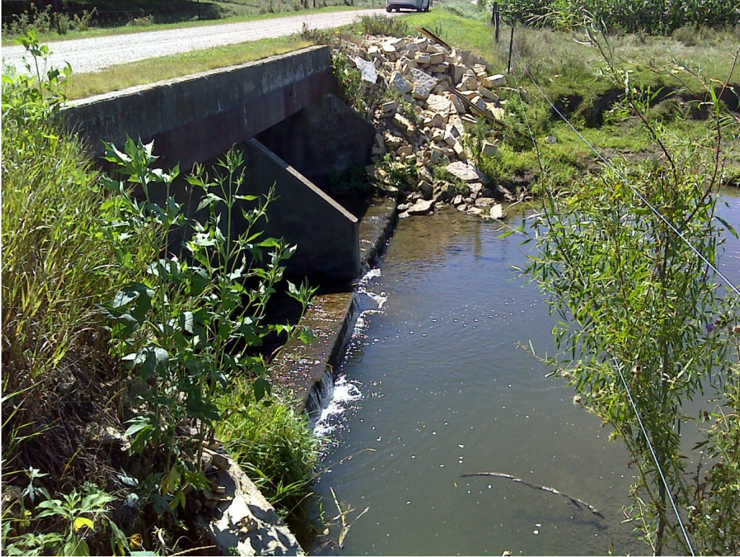
Figure 60. Perched culvert above AUID on 63 rd Avenue.
