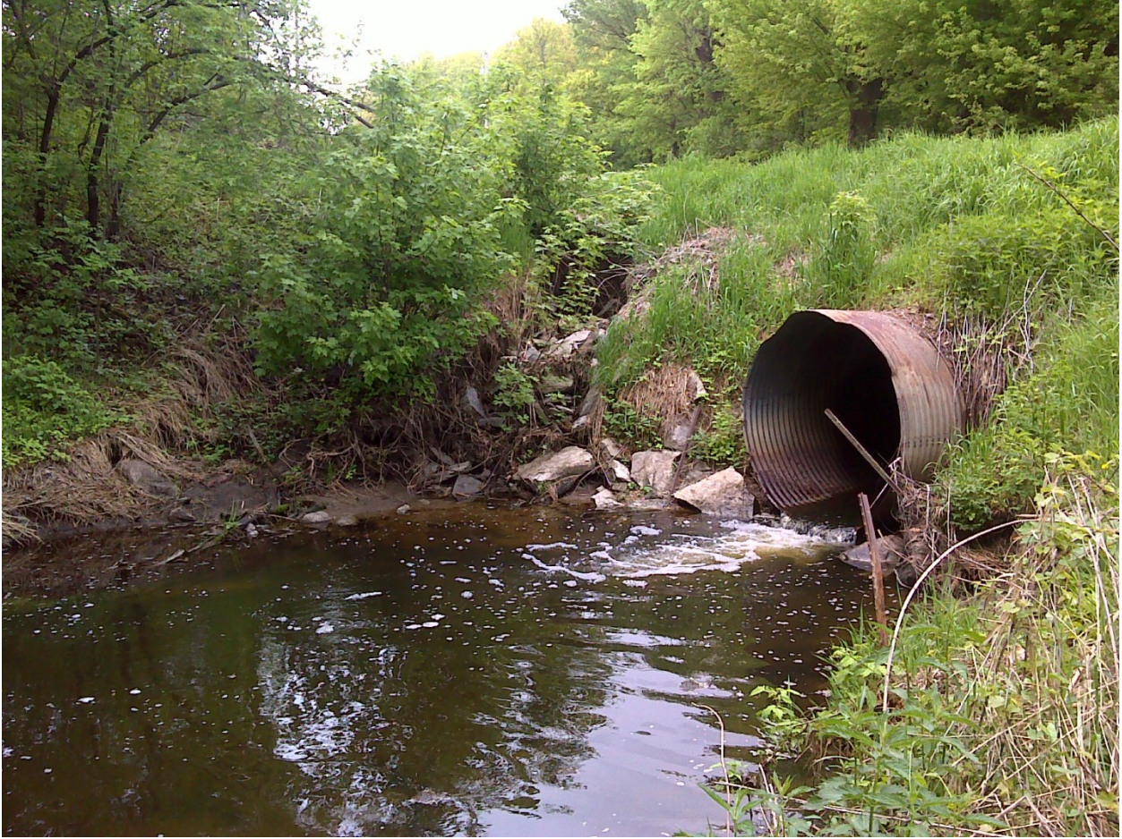
Figure 177. Perched culvert downstream of Union Lake Trail
