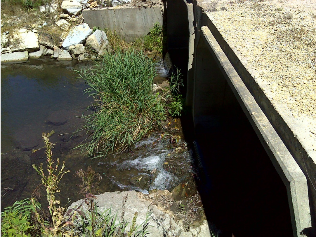
Figure 61. Perched culvert above AUID on 408 th Street Way.
