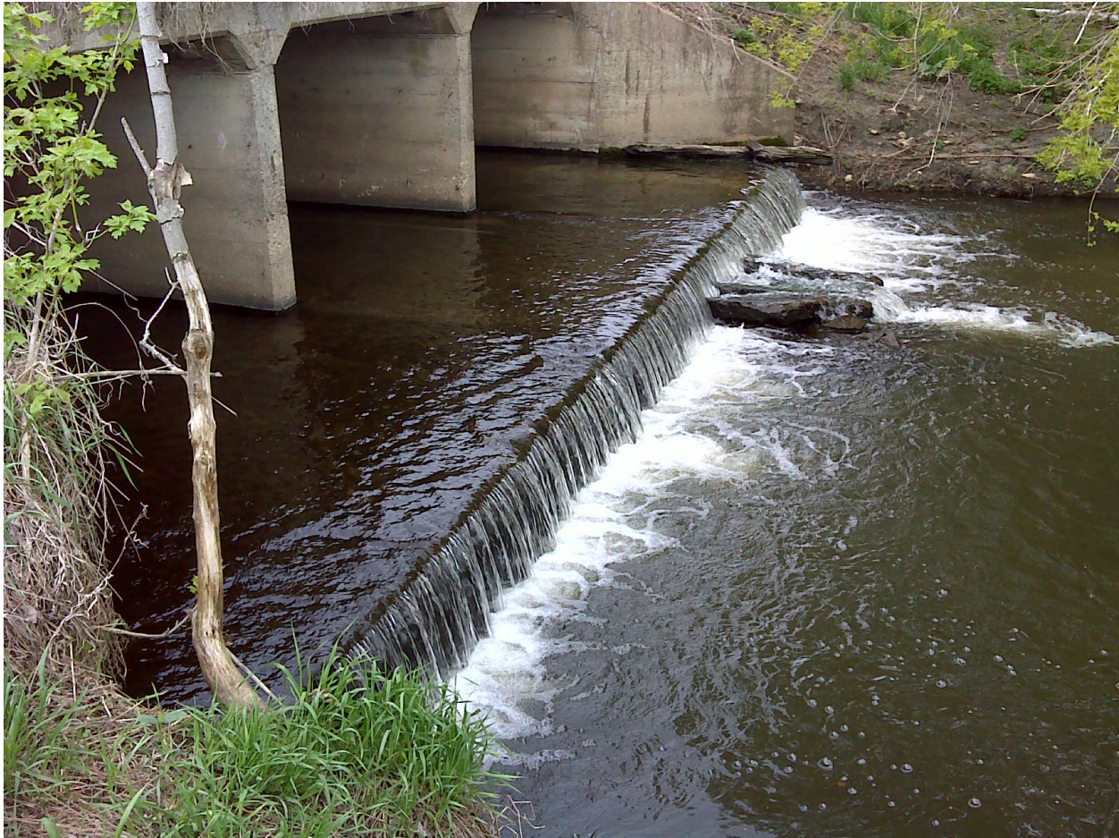
Figure 197. Perched culvert at 23rd Avenue
