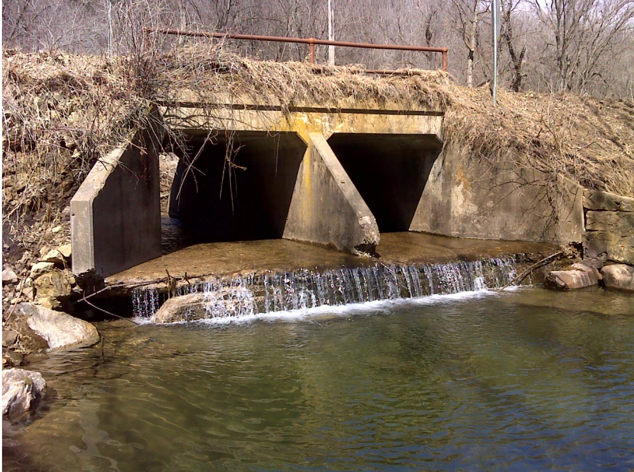
Figure 101. Photograph of perched culvert downstream of Miesville Trail., near station 04LM144 (April 8, 2014)
