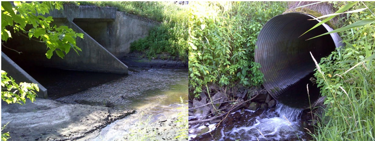
Figure 76. Station S001-245 (Kane Avenue) (left) and 180 th Street (right) during connectivity survey.
